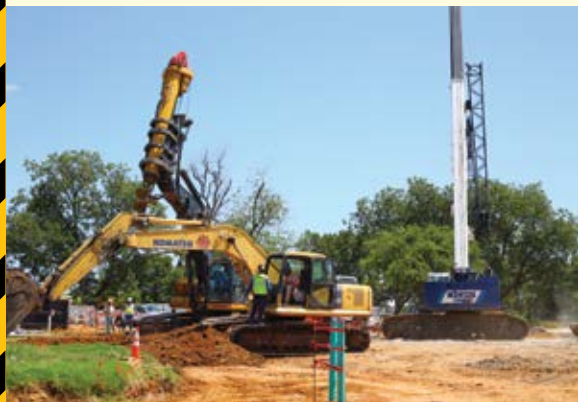
Excavator and pier-drilling equipment on site. The excavator installed two-inch domestic water service.
