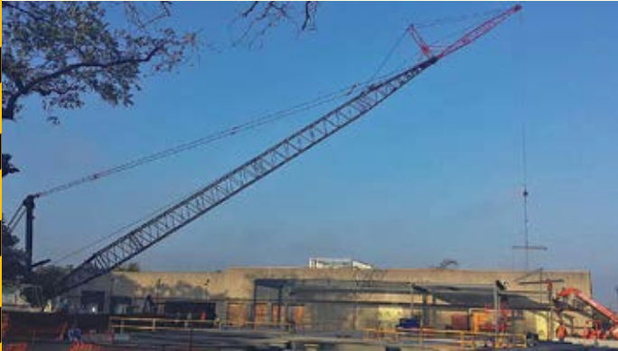
The crane arrived during the last week of October to erect steel beams.
